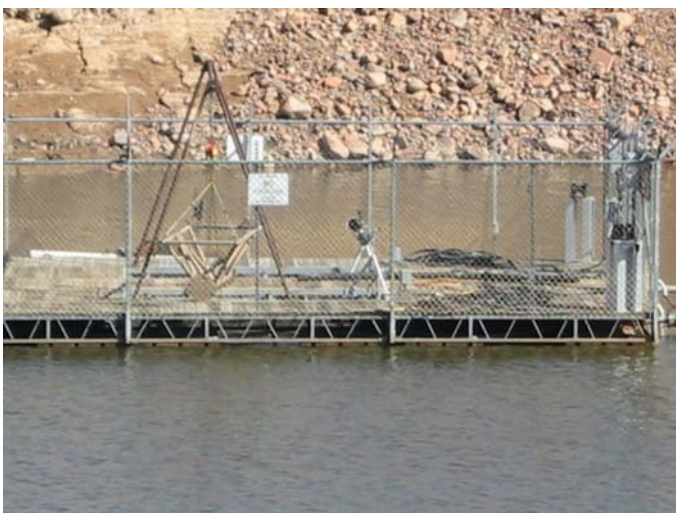
Lake Intake Structures Floating (left) and Stationary (top)
