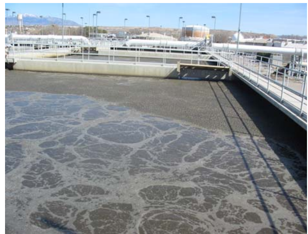
Denitrification Basin Final Aeration Stage
