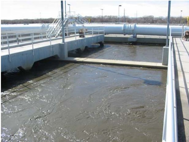
Denitrification Basin Anoxic Stage
