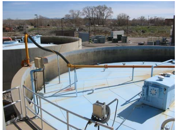
Secondary Digester with Floating Cover
