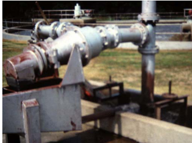
Grit is separated and deposited in a grit classifier (left side) and the water is returned as a sidestream (right side).
